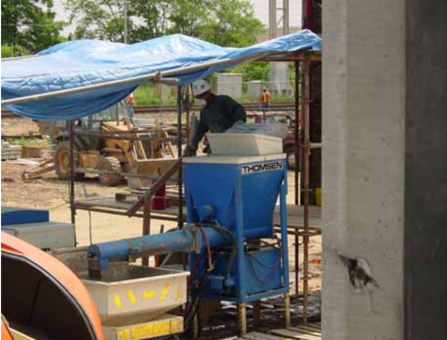
The job was sprayed with a Thomsen Big Blue with a continuous mixer set up. With 600 feet of hose length required the material pumped well at low pressures.
