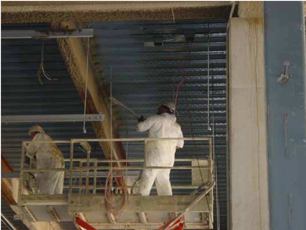
With ceiling heights close to 30 feet the entire floor areas needed to be sprayed from a scissor lift.
