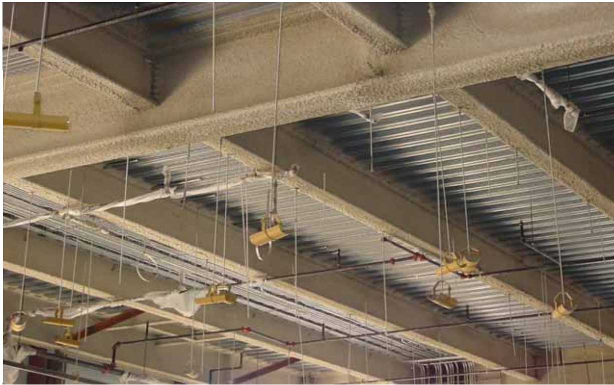
The need for a fine spray textured finish, high bond strength and long term durability made Southwest Type 7GP an excellent choice for the exposed beams and columns throughout the project. No overspray was allowed on the metal decks.
